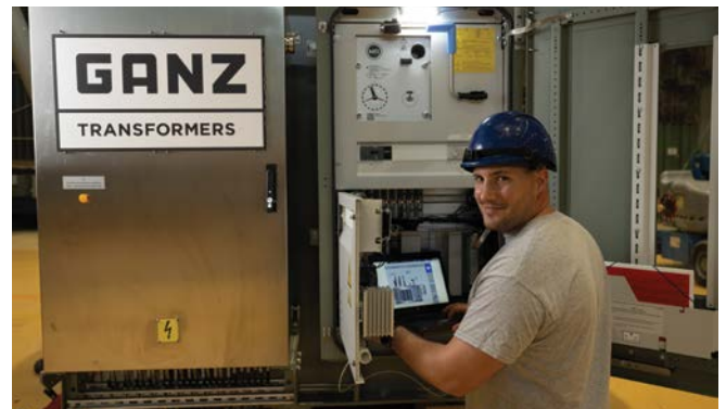
Uncomplicated and fast: With the help of engineering plans, the trained specialists at GANZ can quickly connect GANZ Intelligent Solutions to their transformer in just a few steps.
